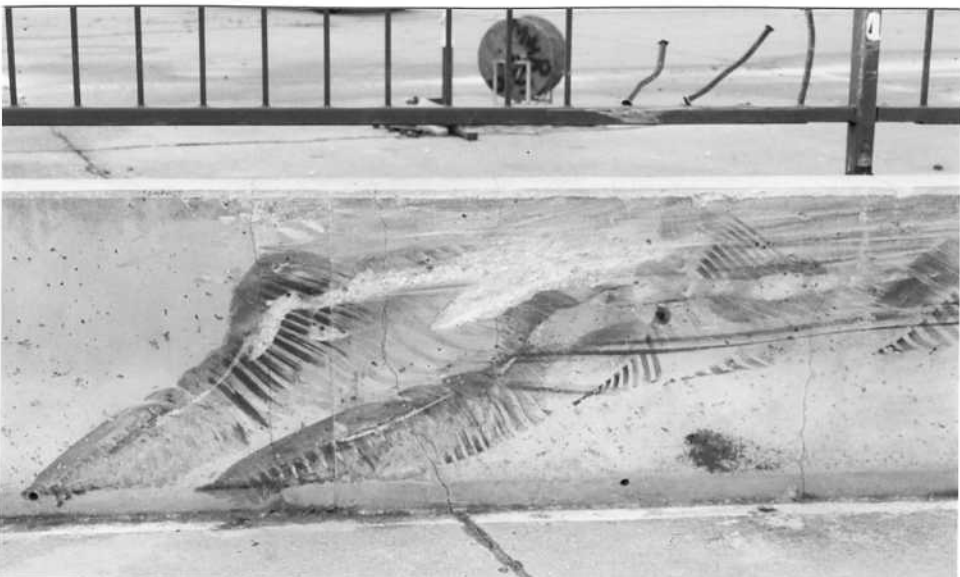
Figure 24. Barrier Damage, Test MNPD-1
