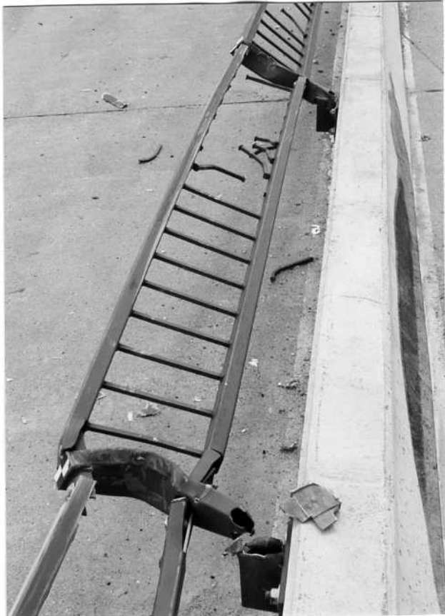
Figure 36. Barrier Damage, Test MNPD-2 (Continued)
