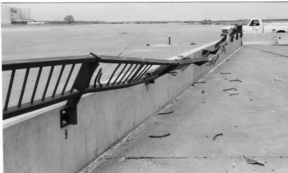
Figure 34. Barrier Damage, Test MNPD-2
