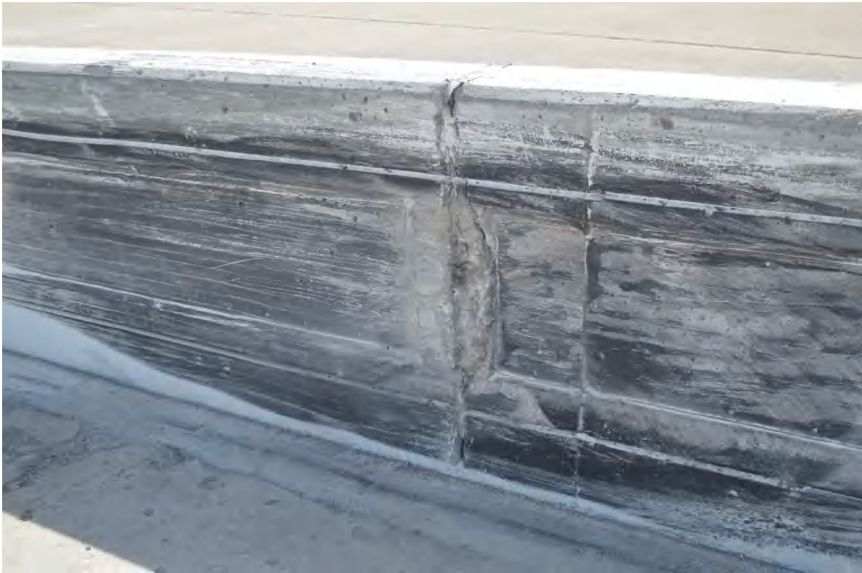
Figure 56. Traffic-Side System Damage, Test No. H34BR-2
